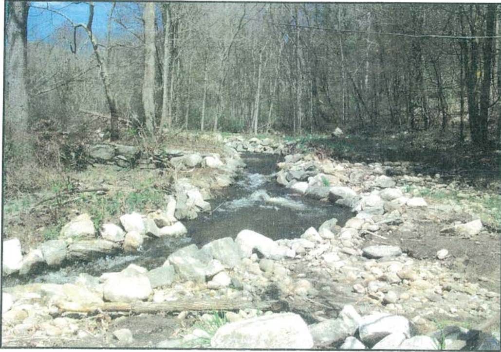
Bypass channel around the Cannondale Dam on the Norwalk River, Wilton.
