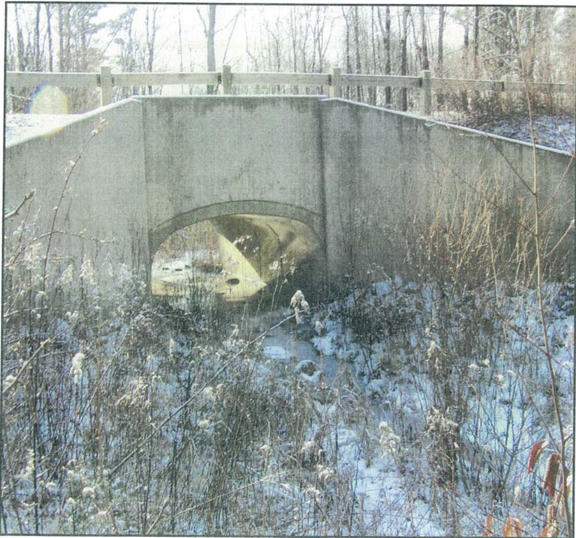
Example of an arch culvert. Road crossing of an unnamed stream at the Litchfield Hollow residential subdivision, Litchfield.
