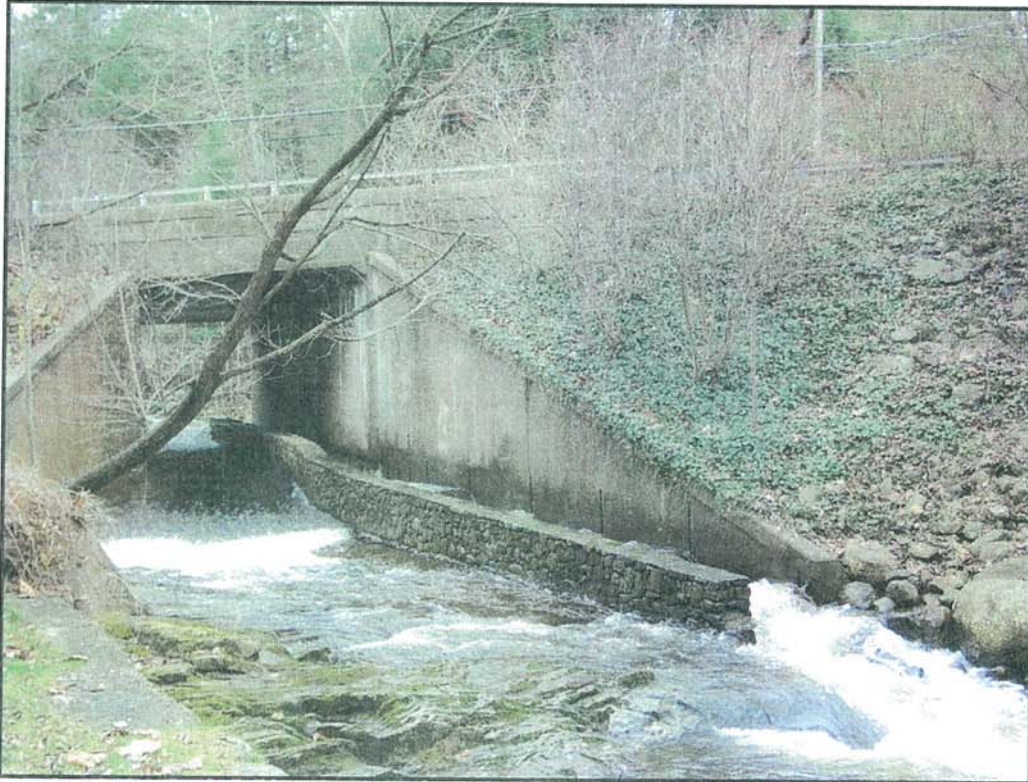
Fishway installed by the Connecticut Department of Transportation at the Route 4 crossing of Furnace Brook, Cornwall Bridge. The fishway was installed to provide passage for brook trout and brown trout.
